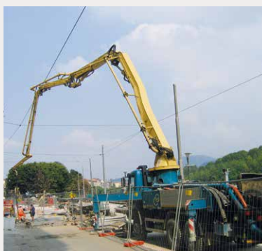
Pompaggio CLS alleggerito a base di Pomical / Pumping of lightened concrete having as basis Pomical
